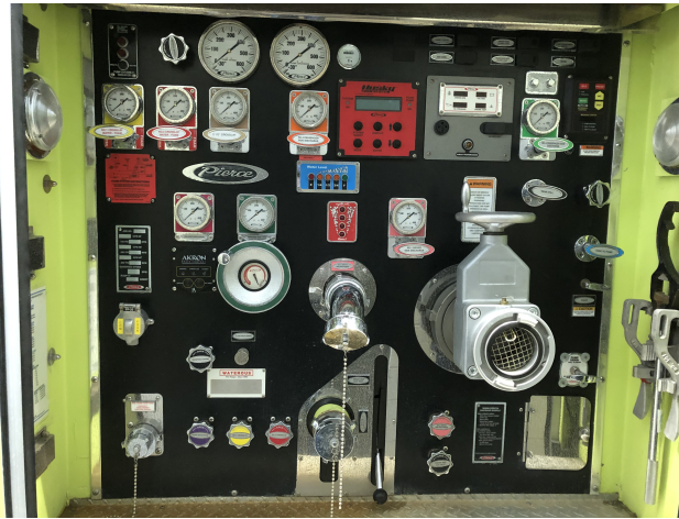
Photo 9: Engine 5 Control Panel
