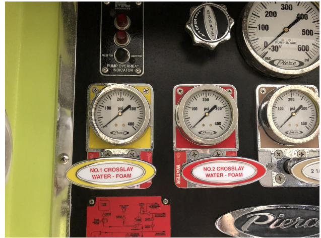
Photo 10: Engine 5 Electric AFFF Proportioner Behind Panel
