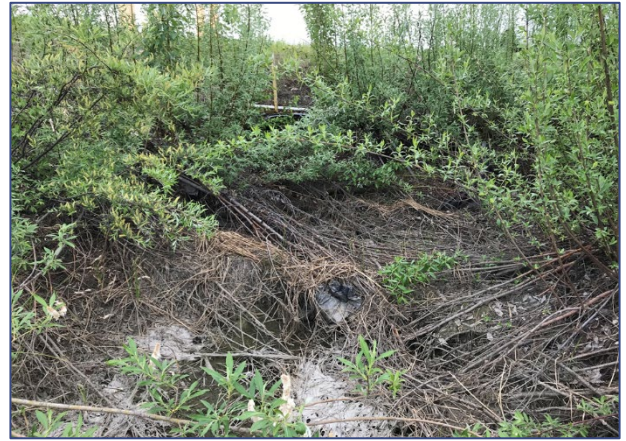
Exhibit 2-1: Condition of the culvert on June 8, 2021
